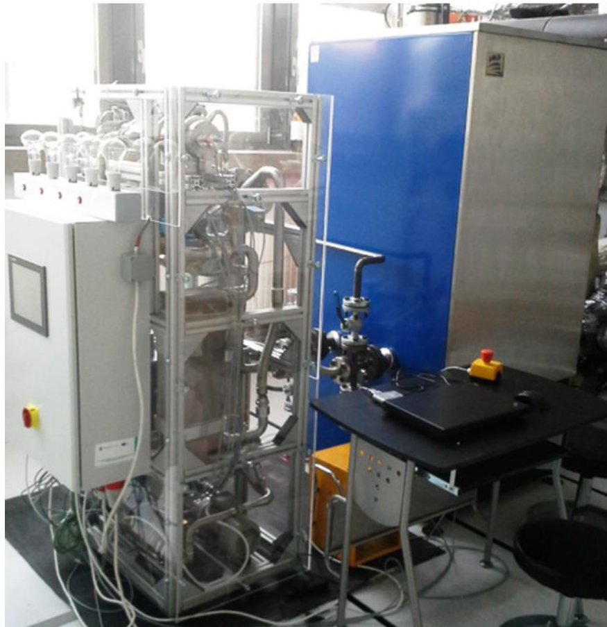
Fig. 2. Photo of the micro ORC power plant.
